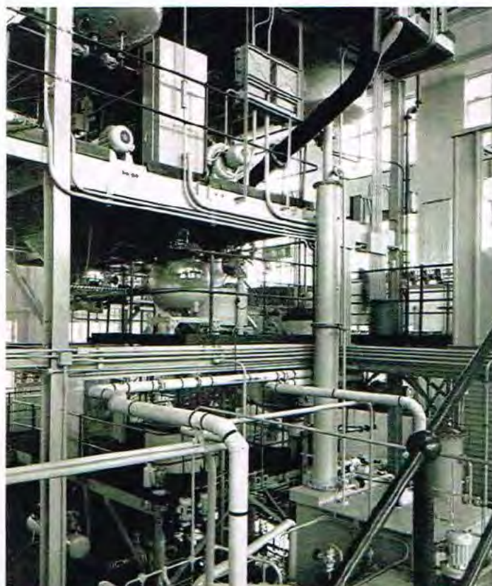
The NCR Emulsion plant at Borehamwood. The plant produced £10,000,000 worth of emulsion
